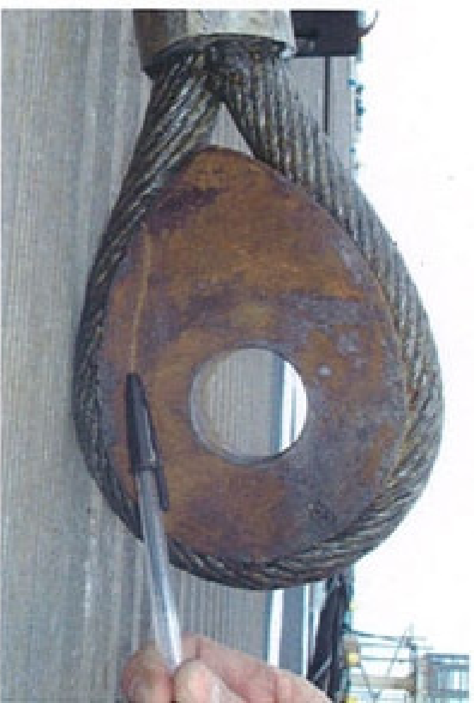
Crack visible on reverse
