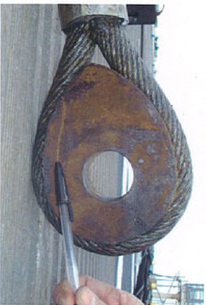
Crack visible on reverse
