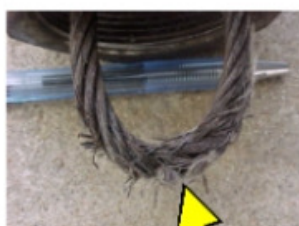
An internal whip-check protection in a poor state of repair – frayed wire.
