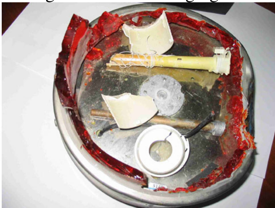
Damaged aircraft warning light
