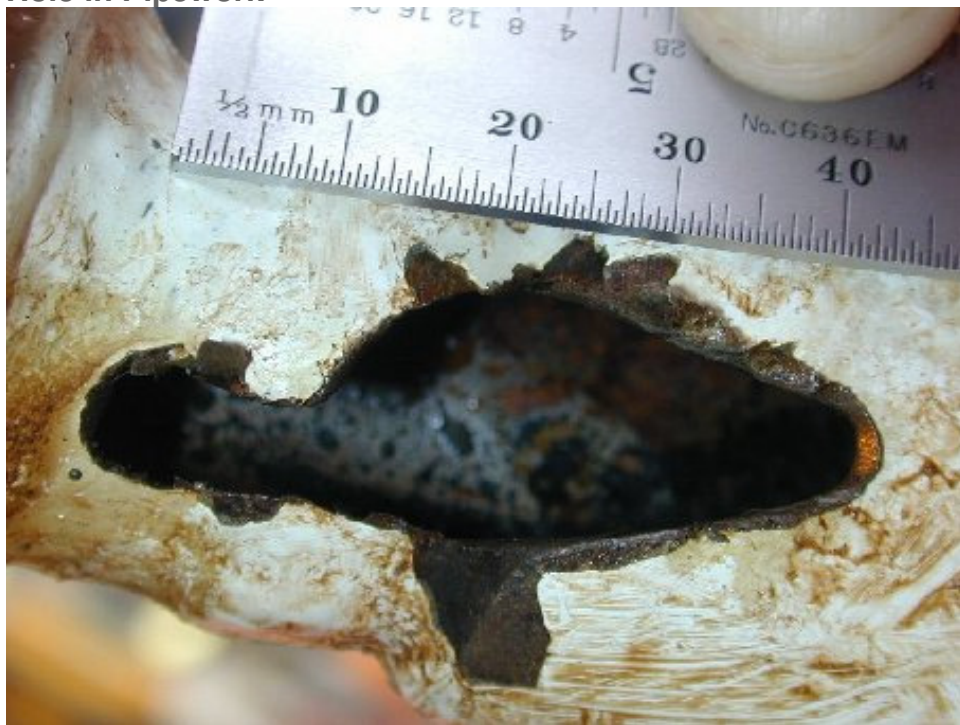
Hole in Pipework
