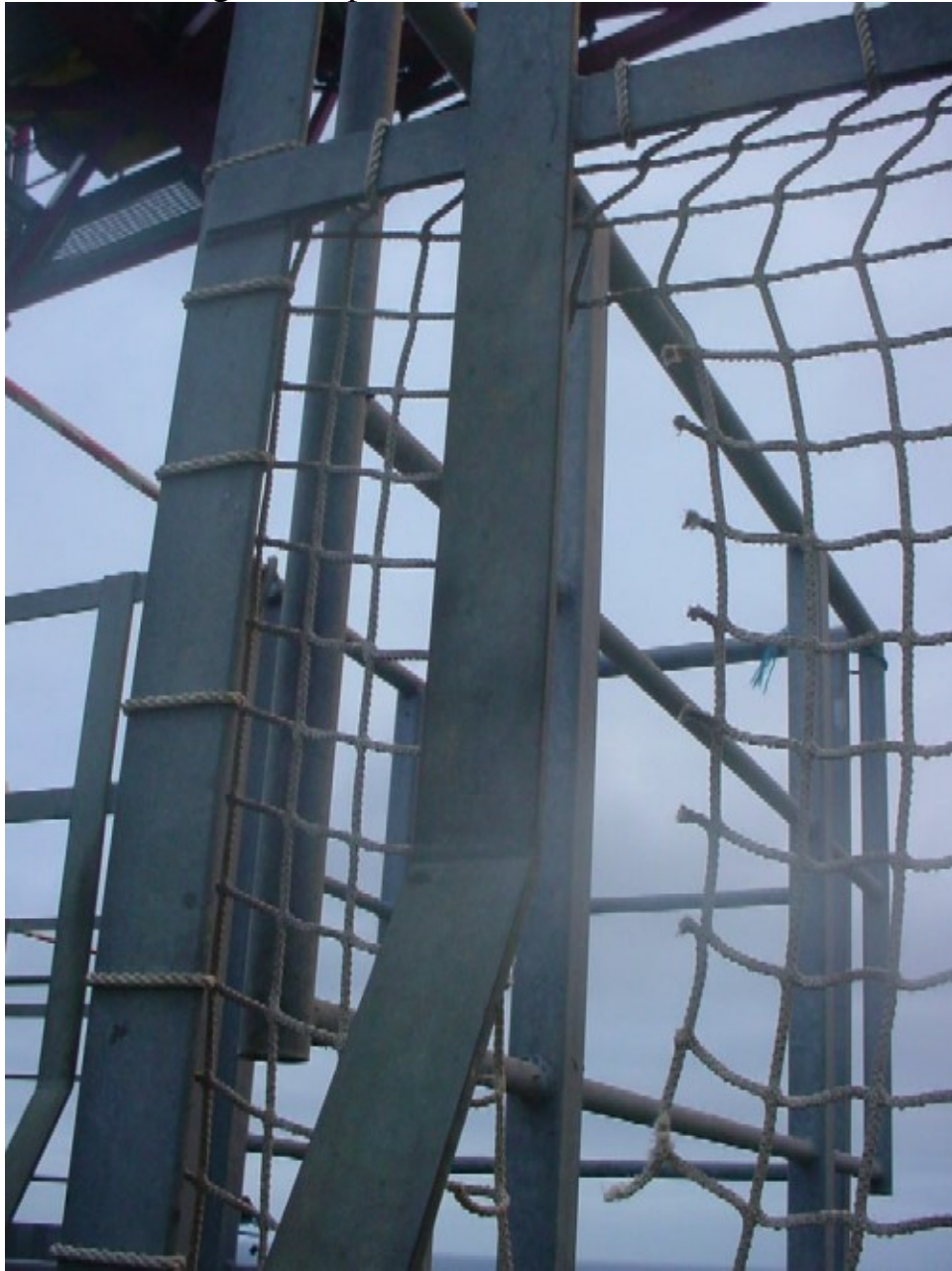
Tear in Netting - Example 2
