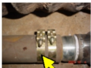
Clamps similar to this were used to hold the flexible airline in place.
