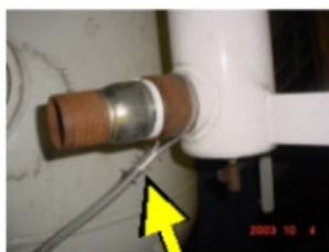
A safety whip-check was installed similar to this.
