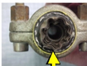
From the photo you can see the use of duct tape to increase the size of the barbed tailpiece.
