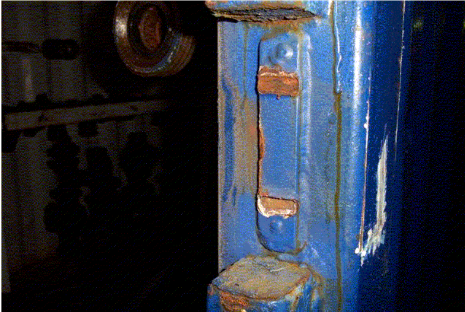
Site of one of the Failed Welds
