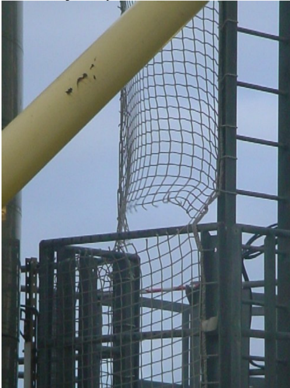
Tear in Netting - Example 1
