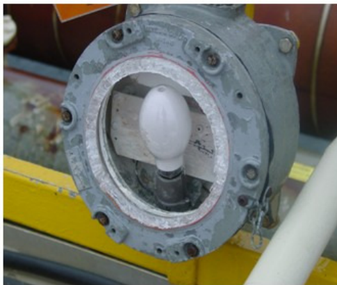
Typical failed fitting
