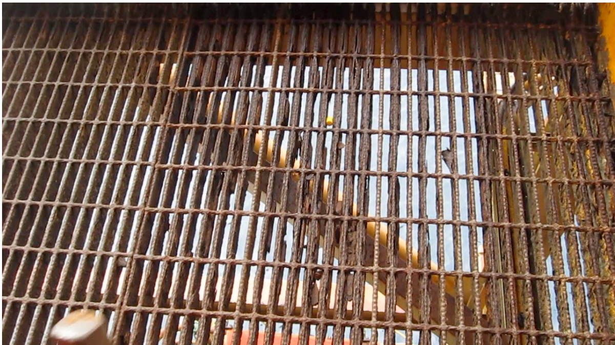
Picture 1: Corroded gratings prior to removal of corrosion product build up
