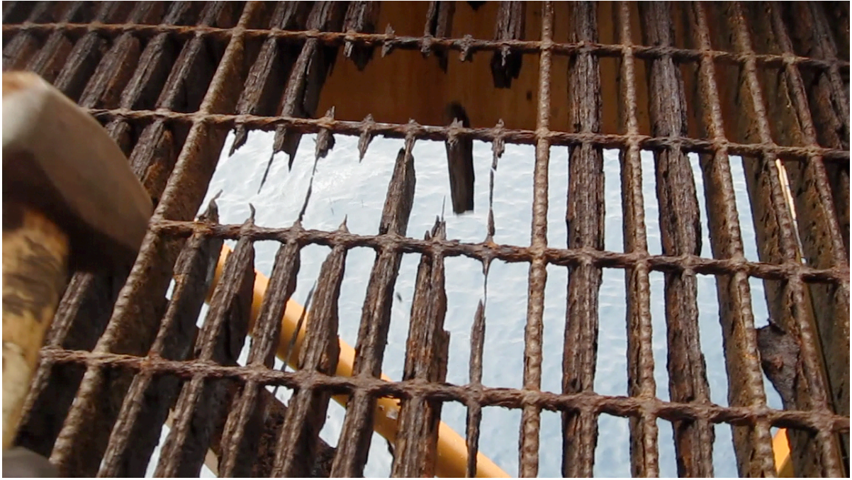
Picture 2: By removing the corrosion product, the severity of metal loss can be seen
