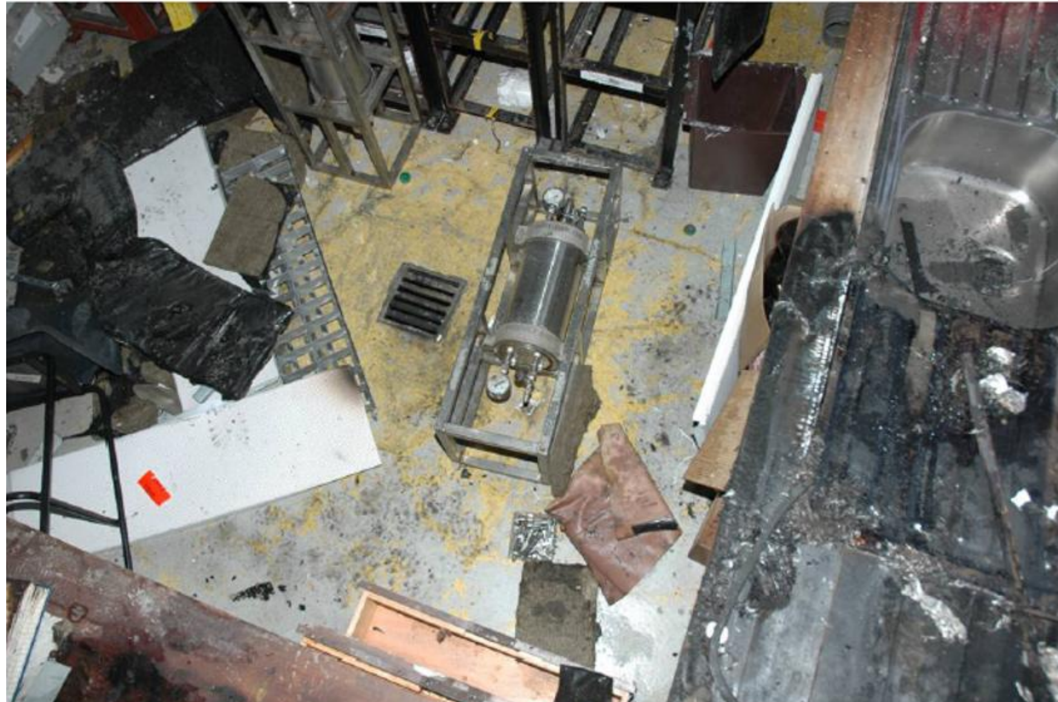
Hydrocarbon source: leaking cylinder and fitting
